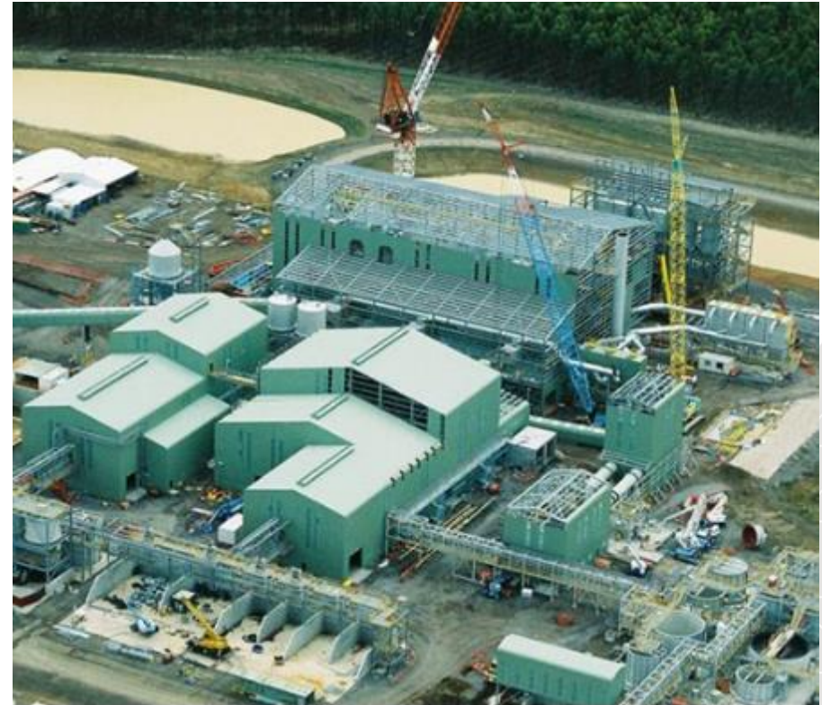
Hamilton Plant, Victoria
