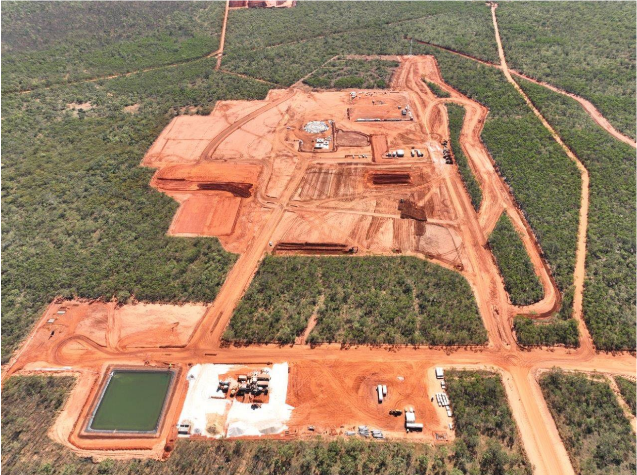
Figure 2: Thunderbird site layout showing Process Plant location (background) and concrete works batching plant (foreground)
