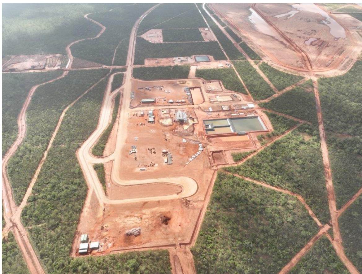
Figure 1: Thunderbird Process Plant site (January 2023)
