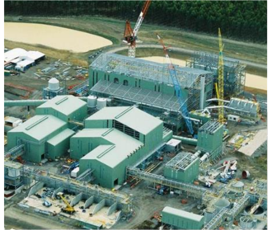
Hamilton Plant, Victoria
