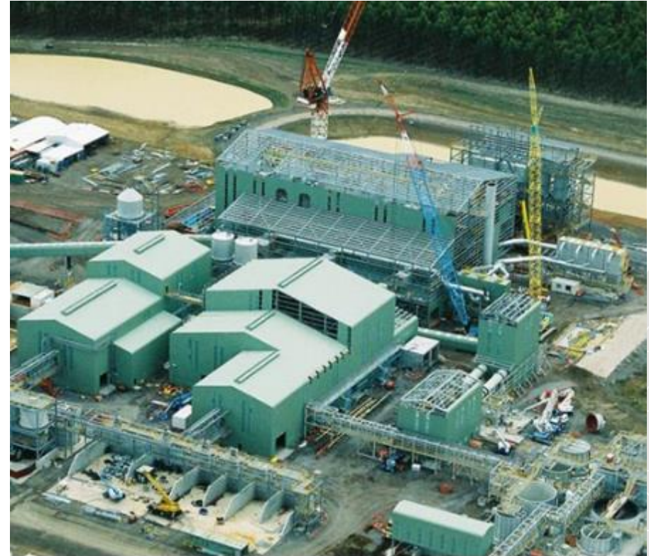
Hamilton Plant, Victoria
